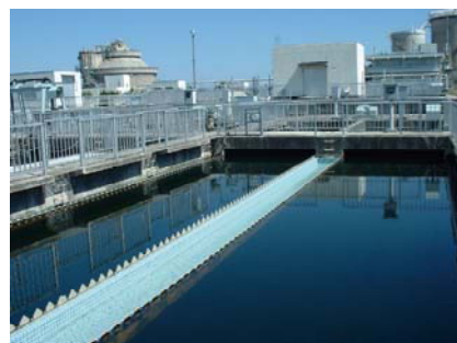
Final Sedimentation Tank
