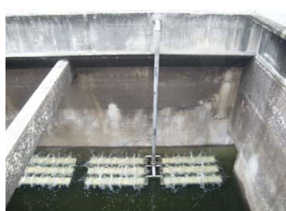
Reaction Tank (Diffuser)
