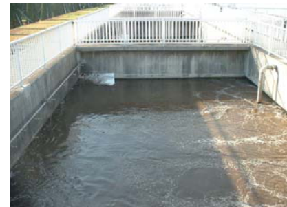
Reaction Tank (Standard Activated Sludge Process)
